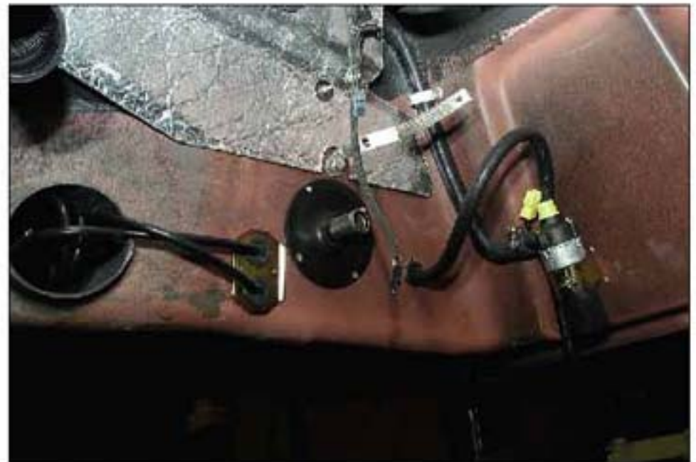
006 RH SIDE VIEW OF LH FUEL TANK CROSS OVER PIPE
