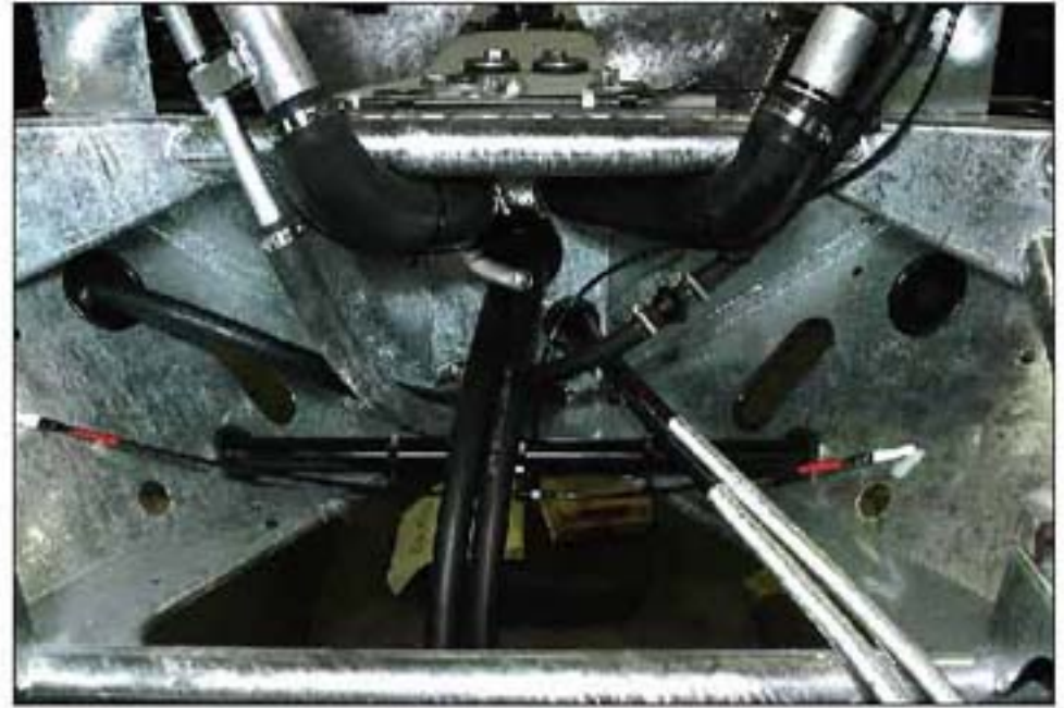
008 CLOSE UP VIEW OF FRONT OF CHASSIS ENG CRADLE
