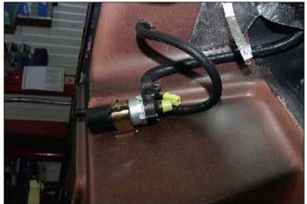
004 RH SIDE VIEW OF COOLING RECIRC PUMP
