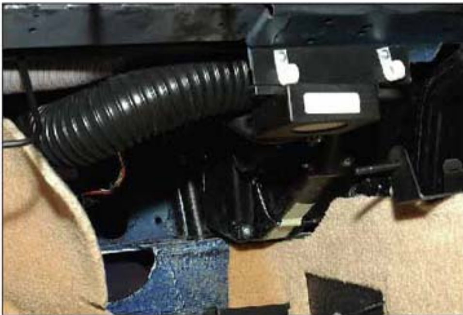
011 REAR LH OBLIQUE VIEW OF HVAC
