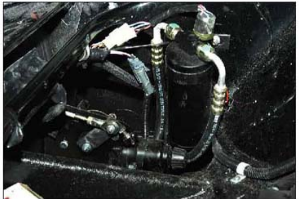
012 VIEW OF RECEIVER DRYER
